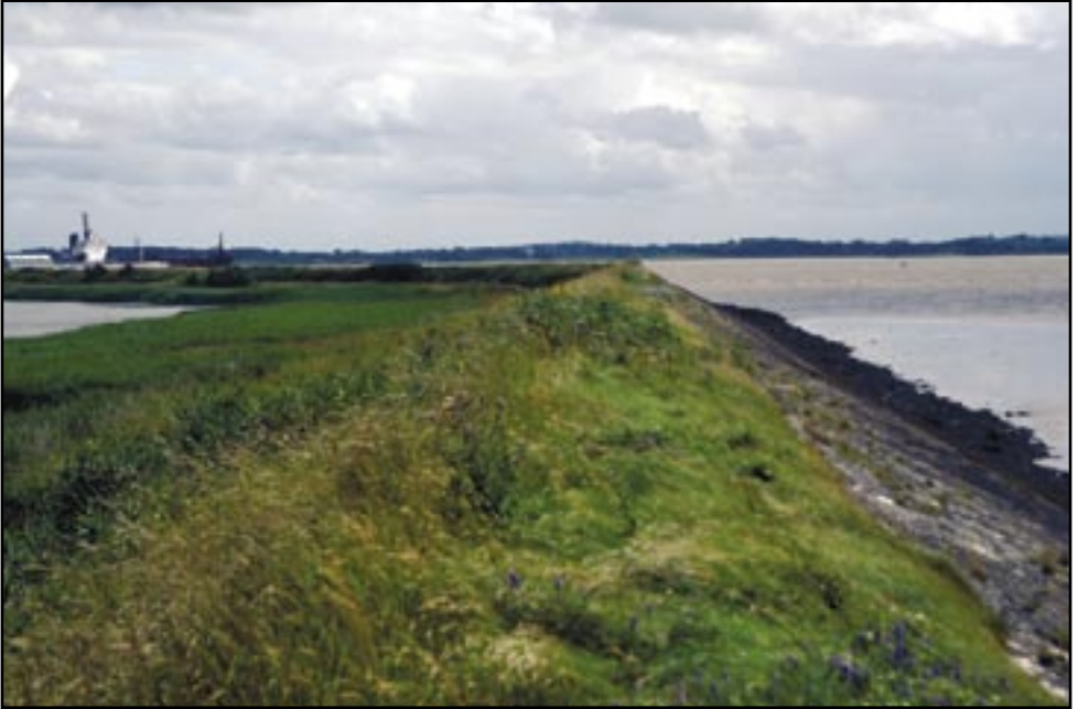
The embankment which helped create the Shannon Airport Lagoon © John N Murphy
